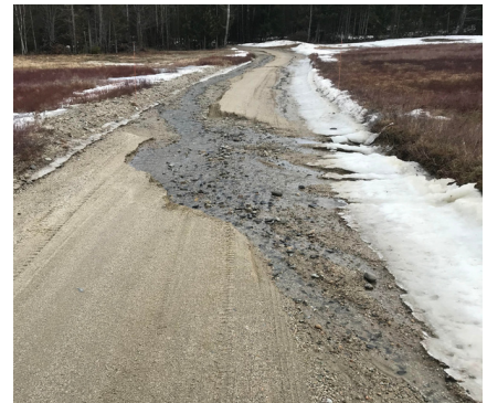
Cousins Road winter 2022 washout
